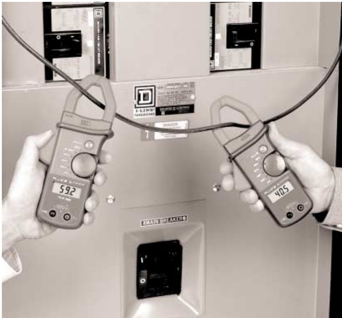
Figure 1 - One current - two readings. Which do you trust? The branch circuit above feeds a non-linear load with distorted current. The True RMS clamp (left) reads correctly but the average responding clamp (right) reads low by 32 %.
