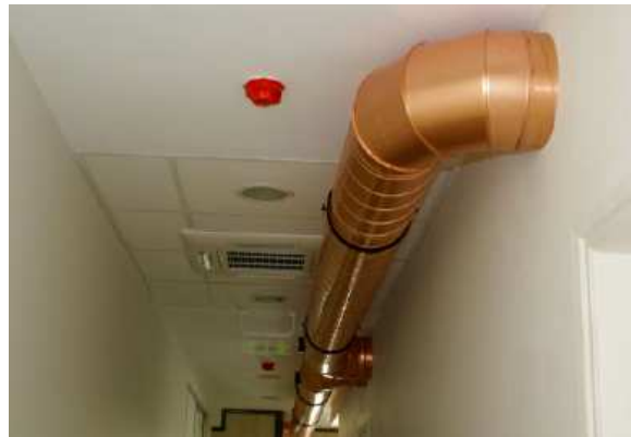
Installed copper ductwork, sidelong
