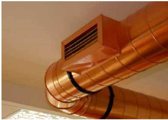
Installed copper ductwork, close up
