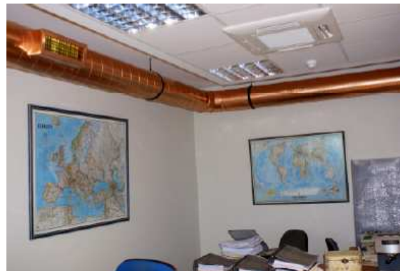
Installed copper ductwork, office interior
