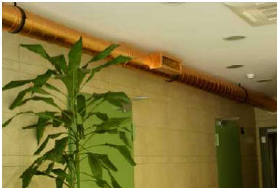
Installed copper ductwork, corridor
