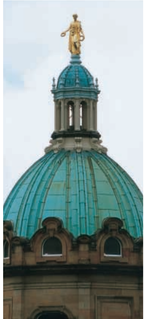
Renovation of top dome, Bank of Scotland HQ, Edinburgh. Roofing Contractor: D. Blake & Co.
