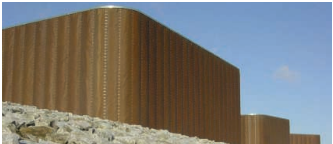
Copper alloy mesh cladding at Plymouth Theatre Royal Production Centre. Architect: Ian Ritchie Architects. Copper Contractors: Lockerwire Weavers/Rubb TM.
